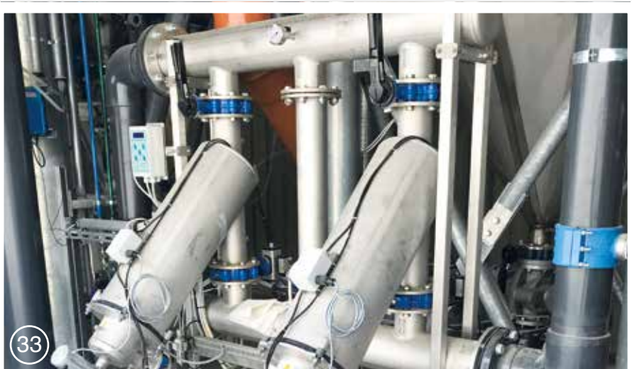
Impianto trattamento acque / Water treatment control panel
